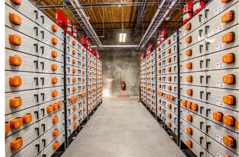
Portland General Electric implemented a multi-service control strategy for the 5 MW/1.25 MWh Lithium-ion ESS at Salem Smart Power Center, Salem, Oregon, USA
